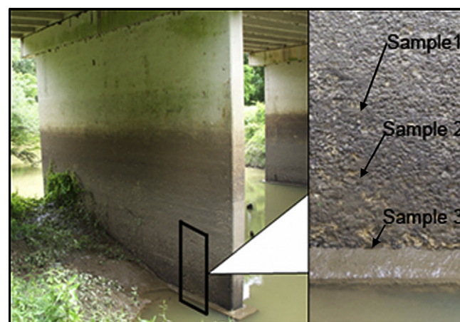
Fig. 1. Bridge support sample sites exhibiting slight (1), moderate (2) and severe (3) corrosion.
